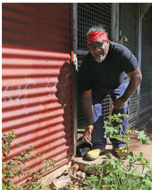
Daniel Palmer pointed out one of many problems with their house in Kalkarindji.
