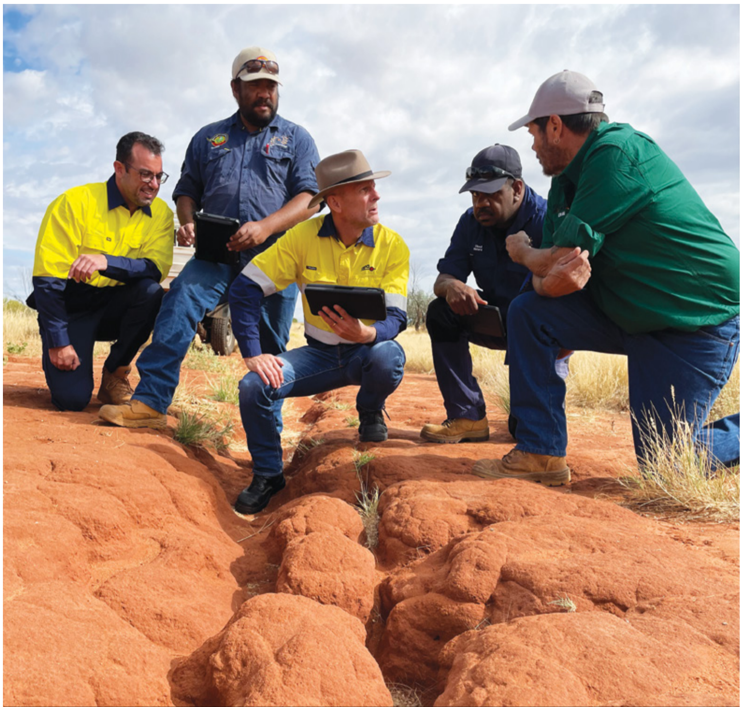
Ben Riley, Cleveland Kantawara, Ross Larsen, Obed Ratarata and Craig LeRossignol inspected some minor erosion along the Amadeus pipeline corridor near Ntaria.
