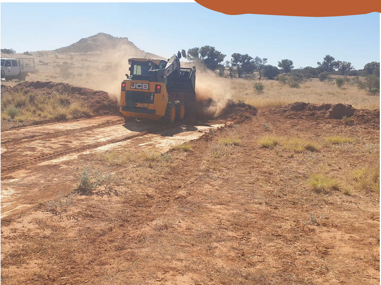
Use of Bobcat to repair erosion control banks on Santa Teresa Land Trust.
