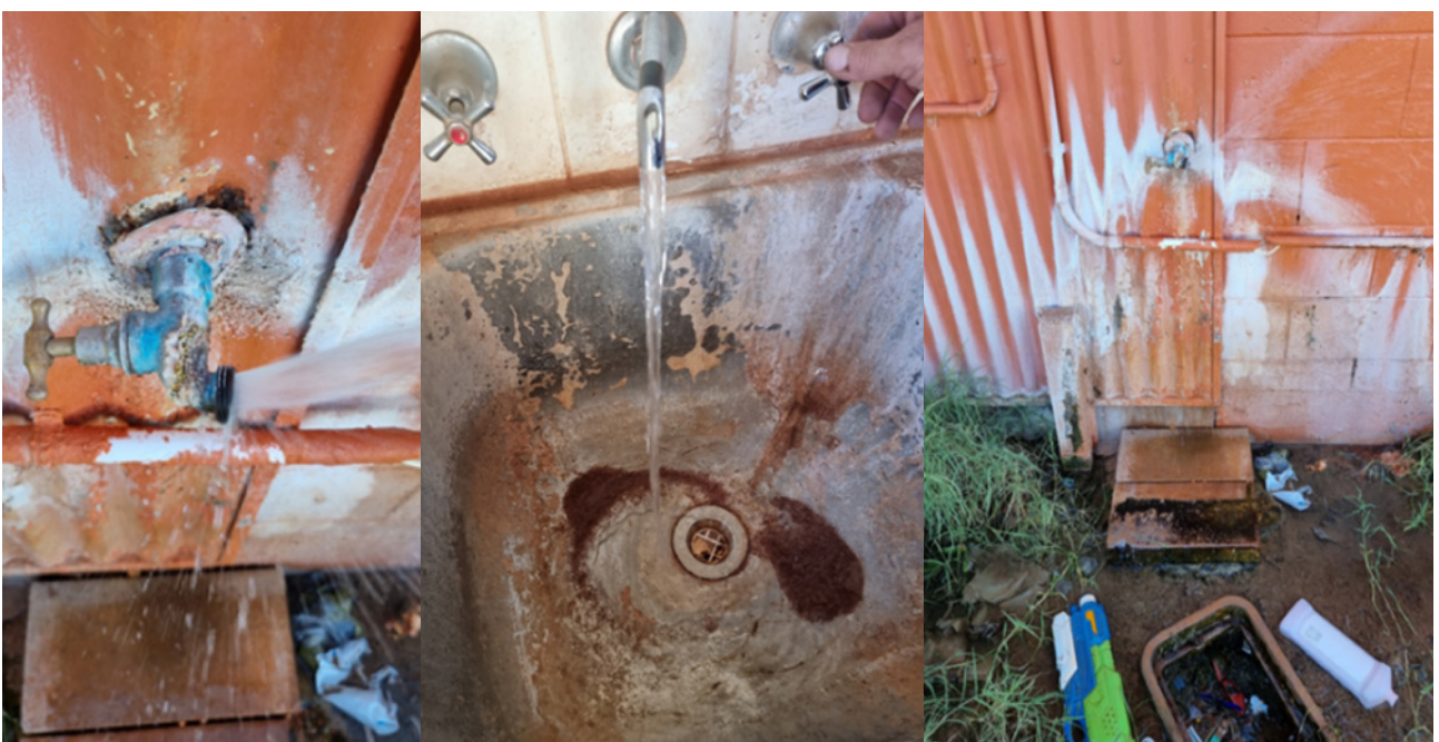
PHOTO 5 Scaling on tap, sink & wall in Alpurrurulam, July 2022
