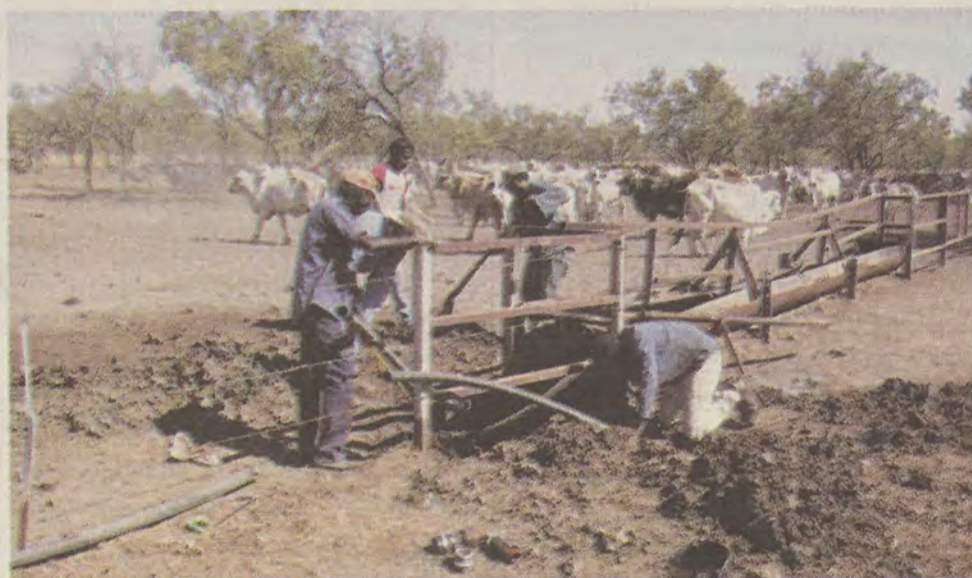
Ngali-Wurru rangers Eric Lewis, Aldrid Jones, Roy MacMillan and Lindsay Daly building a trough at Auvergne Station
