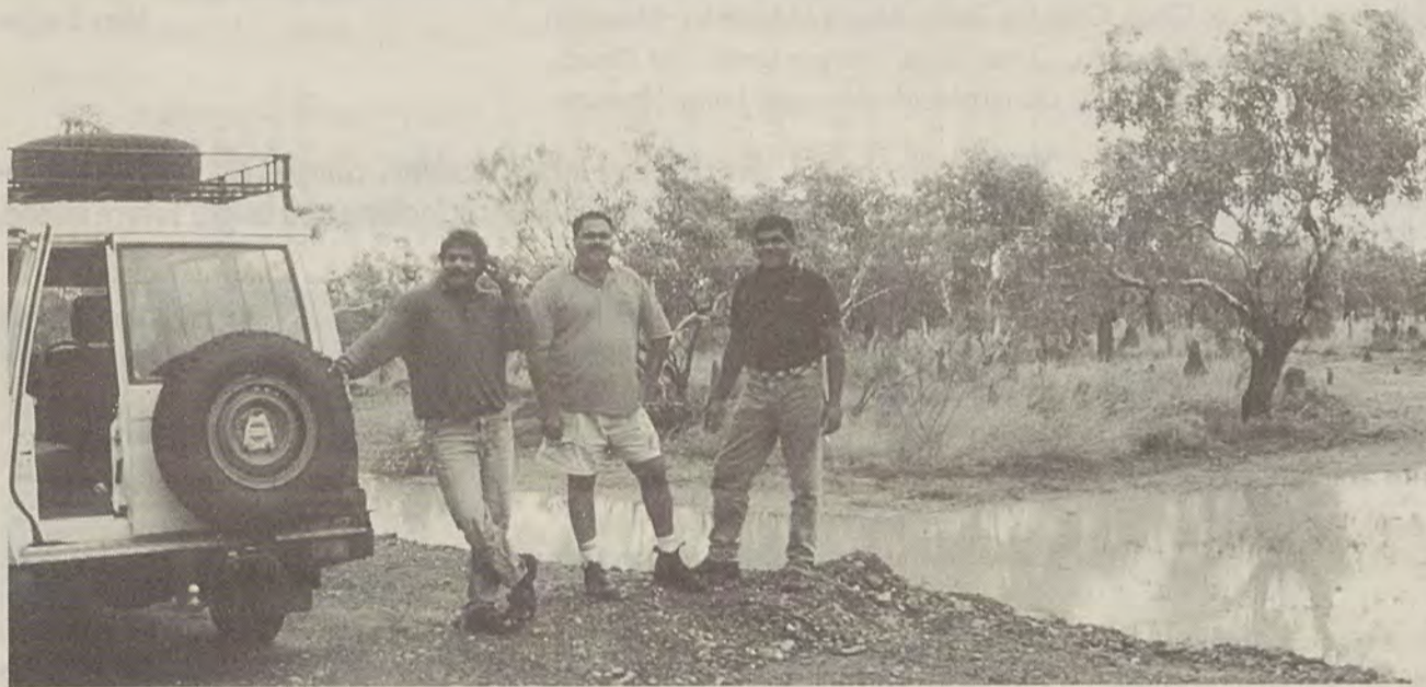
CLC's Tennant Creek staff Ronald Plummer and Brenden Wyman with Norman Frank inspecting a new culvert through a swamp on the access road to Edna Beryl mine. The road has been upgraded as part of the new operation.
