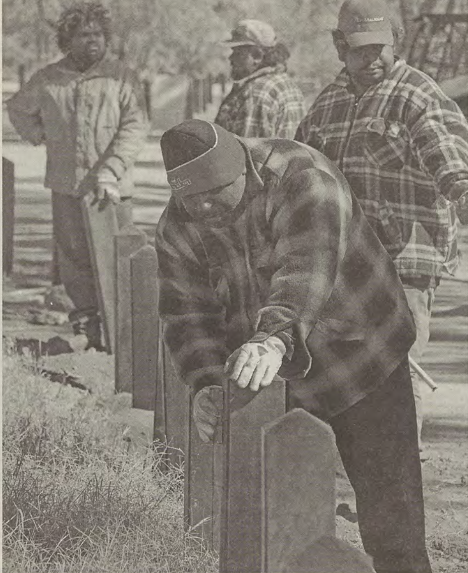
Rangers at work on a contract installing bollards for Parks and Wildlife at Palm Valley this year.
