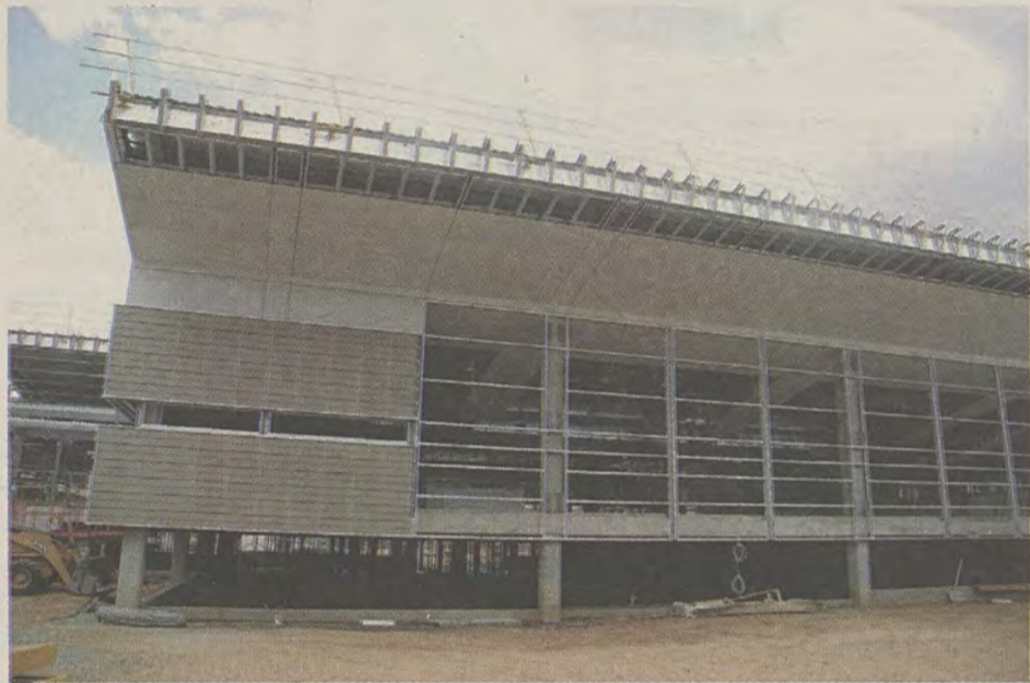
The north side of the new office while it was still under construction late last year.
