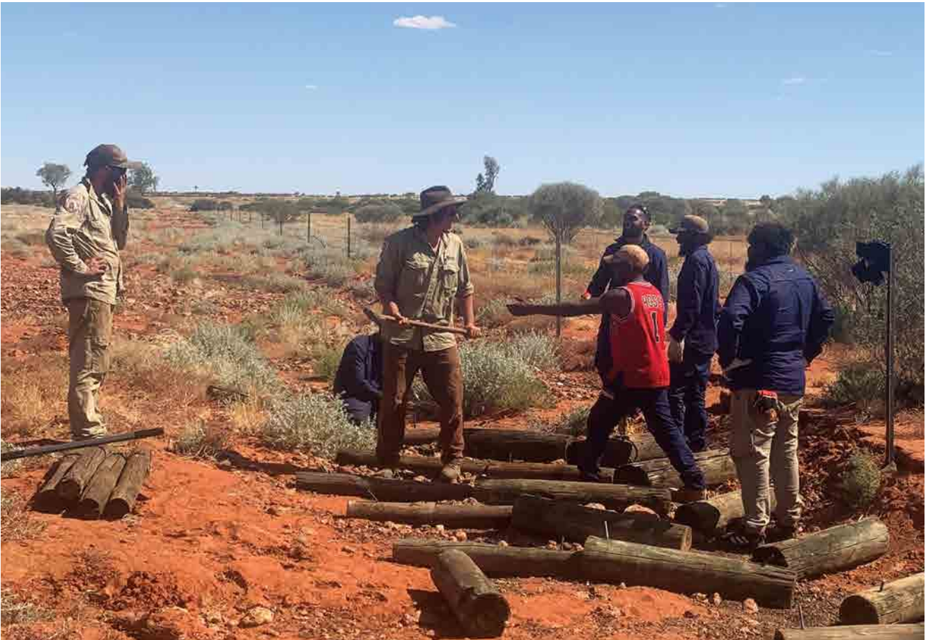
Josh Vartto and Tom Leather (Parks and Wildlife) work with Darren Doolan, Noah Ferguson, Gary Hayes and Barney Jack (Aputula Rangers) to remediate erosion on Mac Clark ( Acacia peuce ) Conservation Reserve.
