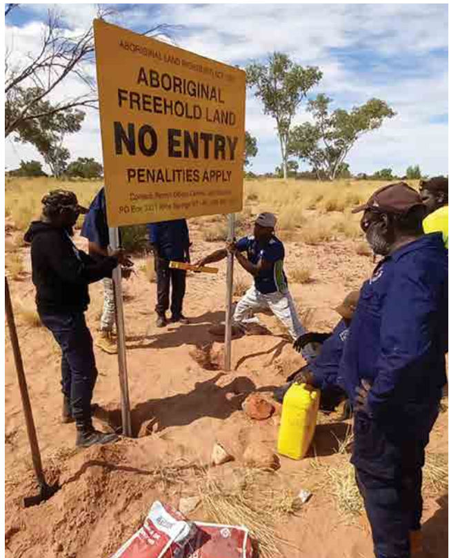
Aputula Rangers installing an Aboriginal Land Trust sign along the Finke Desert Race Track
